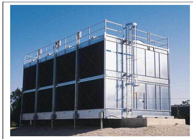
Figure 15 - Induced Draft Cooling Tower
